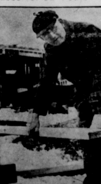
The team of Carrie, 70, and Clarence H. Kessler, 73, has been building homes since their marriage 52 years ago. Here they work on a new house for John Bolewo at Brookfield, Wis. their fifth in the past six years.
