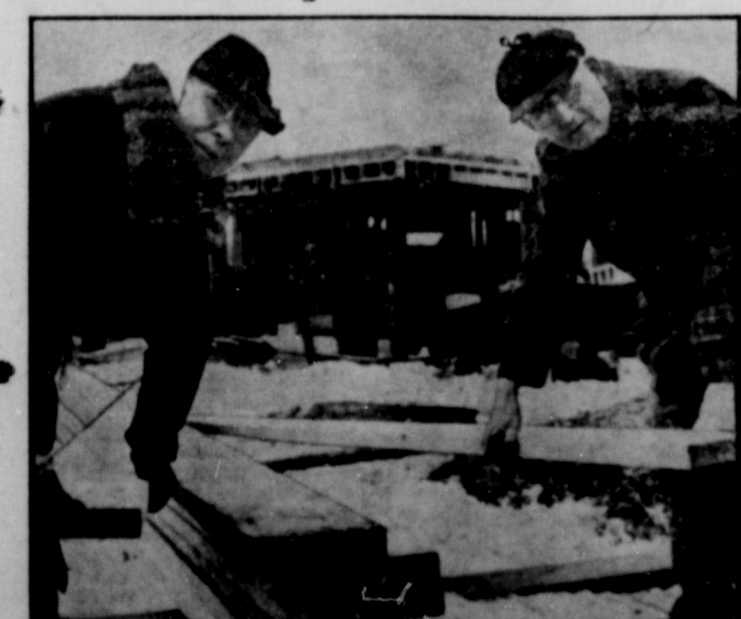
The team of Carrie, 70, and Clarence H. Kessler, 73, has been building homes since their marriage 52 years ago. Here they work on a new house for John Bonome at Brookfield, Wis., their fifth in the past six years.
