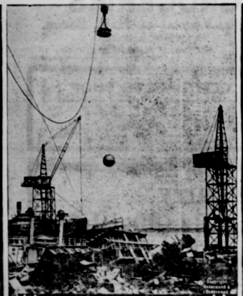
This interesting photograph shows how United States ships which have been sold for junk are being smashed to smithereens in a few minutes at the yards of the Western Marine and Salvage company at Alexandria, Va. The large ball is raised to a height of 75 feet by a huge electro-magnet, and then when the current is cut off the two tons of steel drops with terrific force, breaking the hulls into fragments of commercial size.
