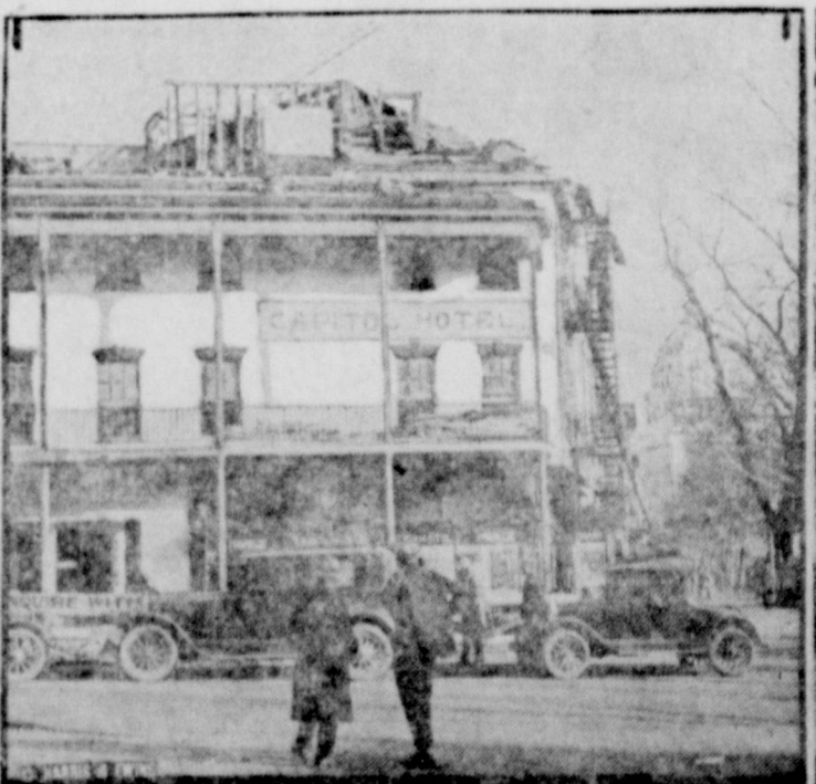
One of the real landmarks of Washington—the old Capitol—here, on Pennsylvania avenue and within a stone's throw of the capitol—is being demolished to make room for a gasoline filling station. The sole surviving relic of slave market days in the national capital, an old auction block, is just north of the hotel.
