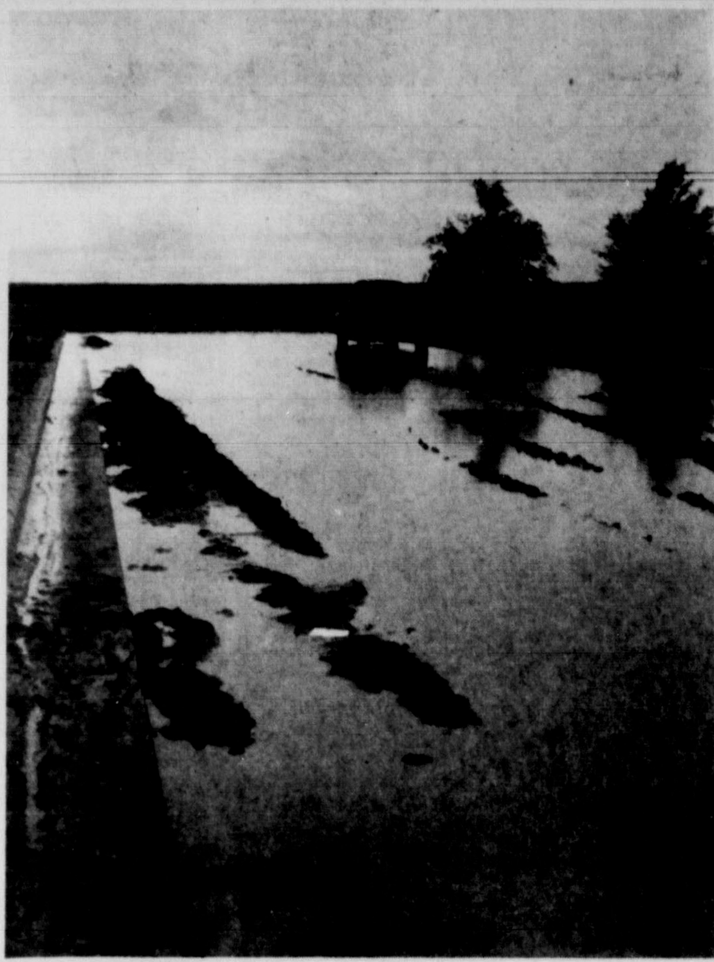
LAKE ASH--Ash Street, one of the streets that run one block off of Fifth Street and under paving looks like a lake Wednesday morning following the rains. Paving crews were busy pumping the water out of the new streets and the bosses were hoping for some sunshine to get things dried out and going again.
