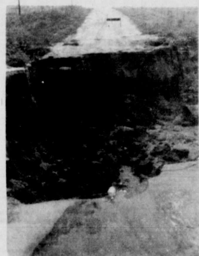
FLOOD WATERS WASHED OUT this road north of the Pleasant Hill community near Frio Draw. The washed-out area was about 15 feet in depth and 30 feet across. This area received nearly 10 inches of rain in one 24-hour period.
