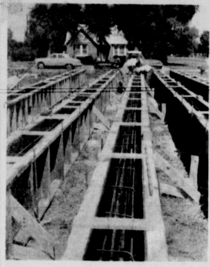
SOMETHING NEW IN FRIONA---As work progresses on the new building which is to house White's Supermarket workmen are shown above fixing forms for the pouring of the concrete beams that will be lifted to form the roof structure of the building. This will be the first structure of this kind to be put up in Friona and the scene attracted many curious onlookers this week.
