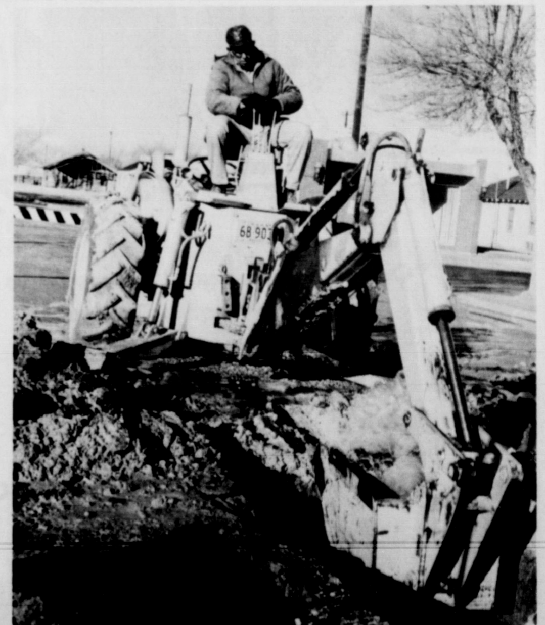
REPAIRING MAIN . . . Friona Water Superintendent Clyde Fields excavates a hole in front of the Post Office, where a four-inch water main burst early this week, a result of the extremely cold temperatures in the city the past few weeks.
