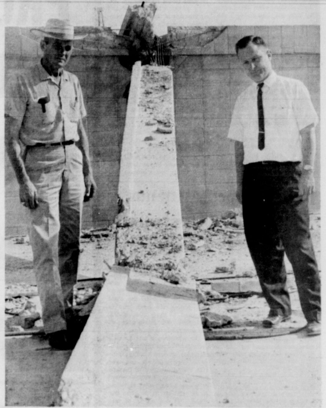
INSPECT DAMAGE . . . George Taylor, contractor, and Joe Gulde of Amarillo inspect the broken cement beam which snapped during a freak accident at the new Johnson Food Market last week.
