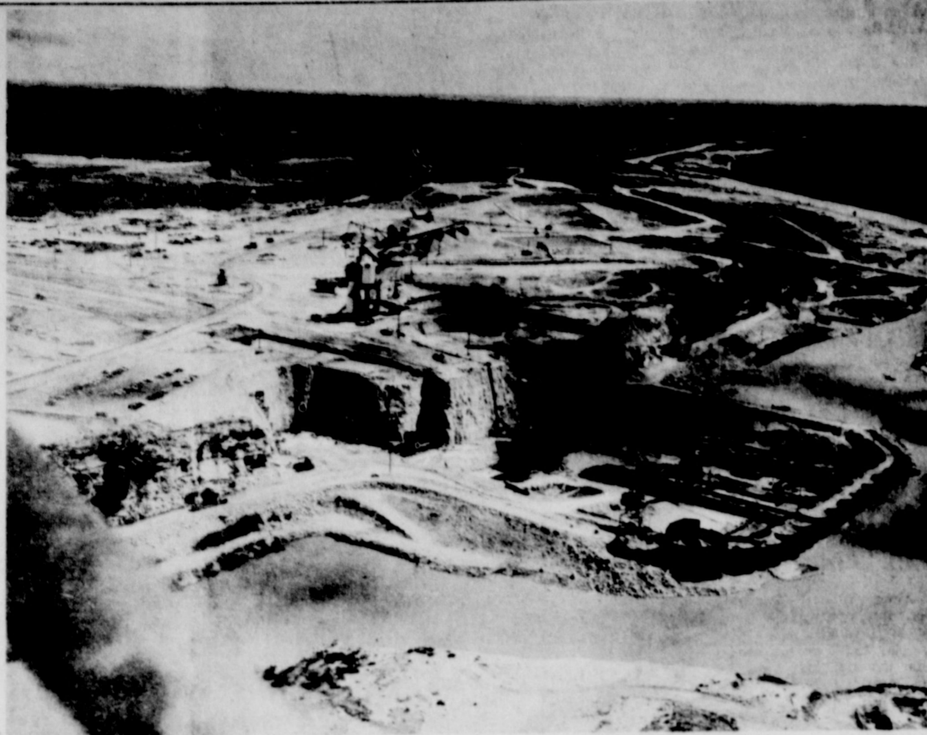
AMISTAD DAMSITE — Only an aerial view of the huge construction project underway astride the Rio Grande can give any conception of Amistad Dam, which will extend six miles and rise 254 feet above the river bed. Located 12 miles upstream from Del Rio, Amistad Dam will impound the waters of the Rio Grande and of Devil's River, backing up 86 miles. Seen in this photo made by James Wardle of the International Boundary and
