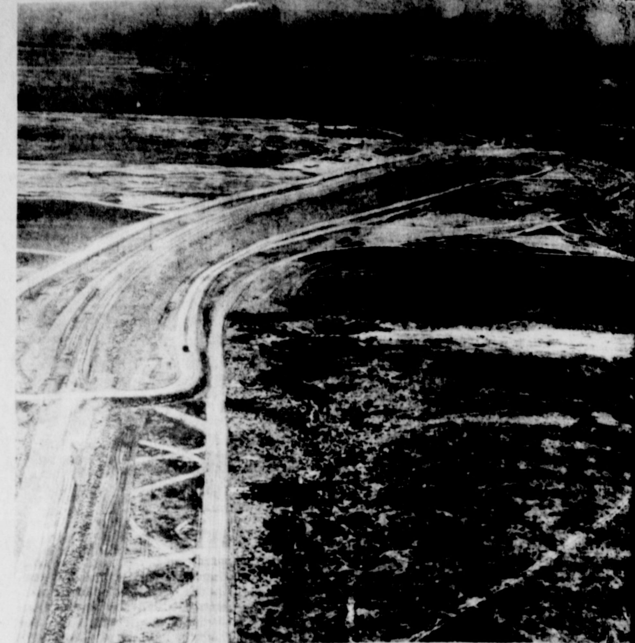
EARTHEN EMBANKMENT — Earthen embankments are constructed on each side of the concrete portion of Amistad Dam, 12 miles upstream from Del Rio on the Rio Grande. This is an aerial view of the embankment on the United States side of the river with the dam itself in the upper right hand corner of the picture. The portion of the earthen embankment in Mexico is almost complete, approximately 98 per cent of that work having been finished. The dam is in the second phase of the construction of the international project. (News-Herald Photo).
