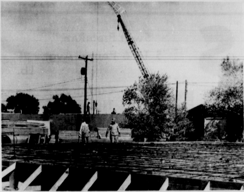
BUSY BLOCK . . . The block bounded by Main and Euclid between 10th and 11th street has a lot of building activity, with the new 10th Street Church of Christ building taking shape in the foreground. In the background, steel beams were being put in place at the construction site of Harry's Super Market.
