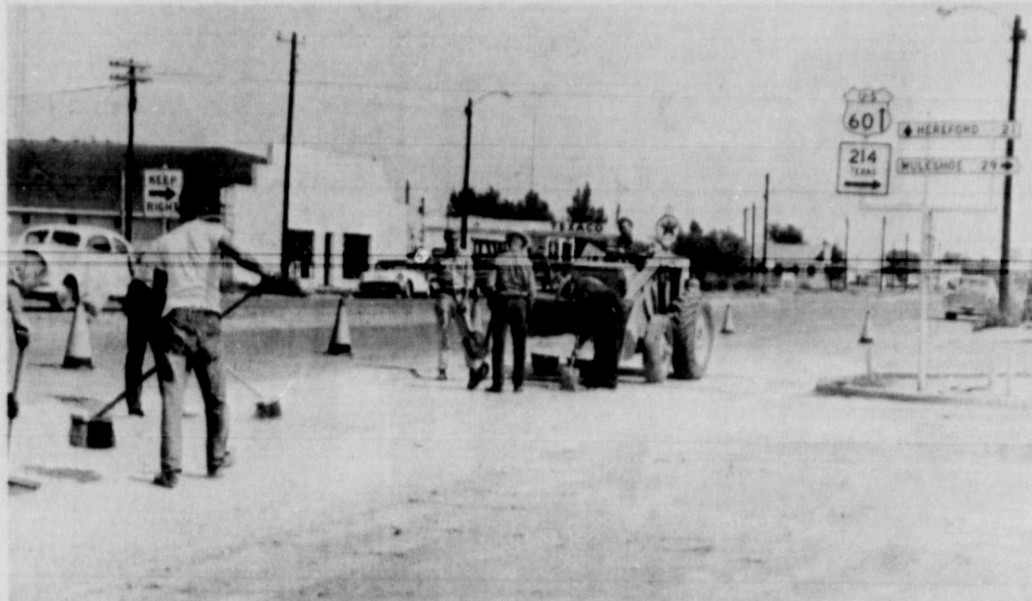
STREET REPAIRS . . . Employees of the Texas Highway Department are caught making repairs on North Main Street in Friona, at the intersection of State Highway 214 and U. S. Highway 60. The intersection easily becomes rough, due to constant traffic and right turns onto Friona's Main Street.
