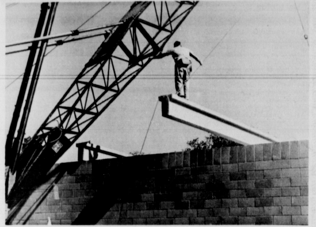
BUILDING PROGRESSES... Pre-stressed concrete beams were put in place at the Spudnut factory which is being built in Friona. The building is progressing nicely. The factory is to be in operation by September 1, and the building is well on schedule.
