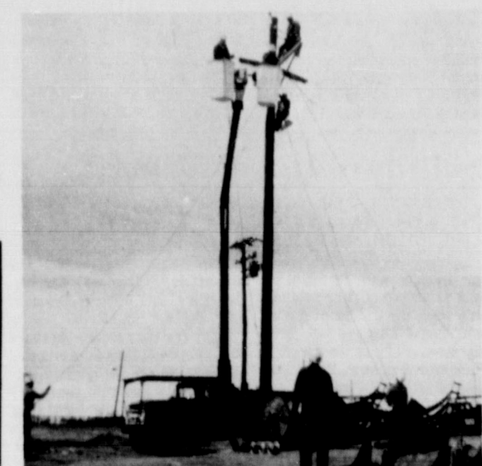
HIGH LINE WORK. . . Work on a 23,000-volt line is being done in this photograph, taken at Third and Grand in Friona. Assisted by a two-man bucket crew, the SWPS work was carried out while the line was "hot".
