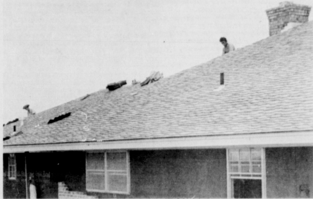
Typical of the construction going on in Friona is the new home currently under construction by R. L. Fleming & Son. The home is being built in one of the city's new additions, Western Addition.
