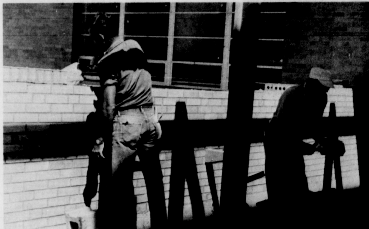
WORKMEN BUSY. . . Workers at the new high school site are working "full steam ahead" in order to get the new facility ready for the opening of school August 30. School officials say that classroom portions of the school will be ready.
