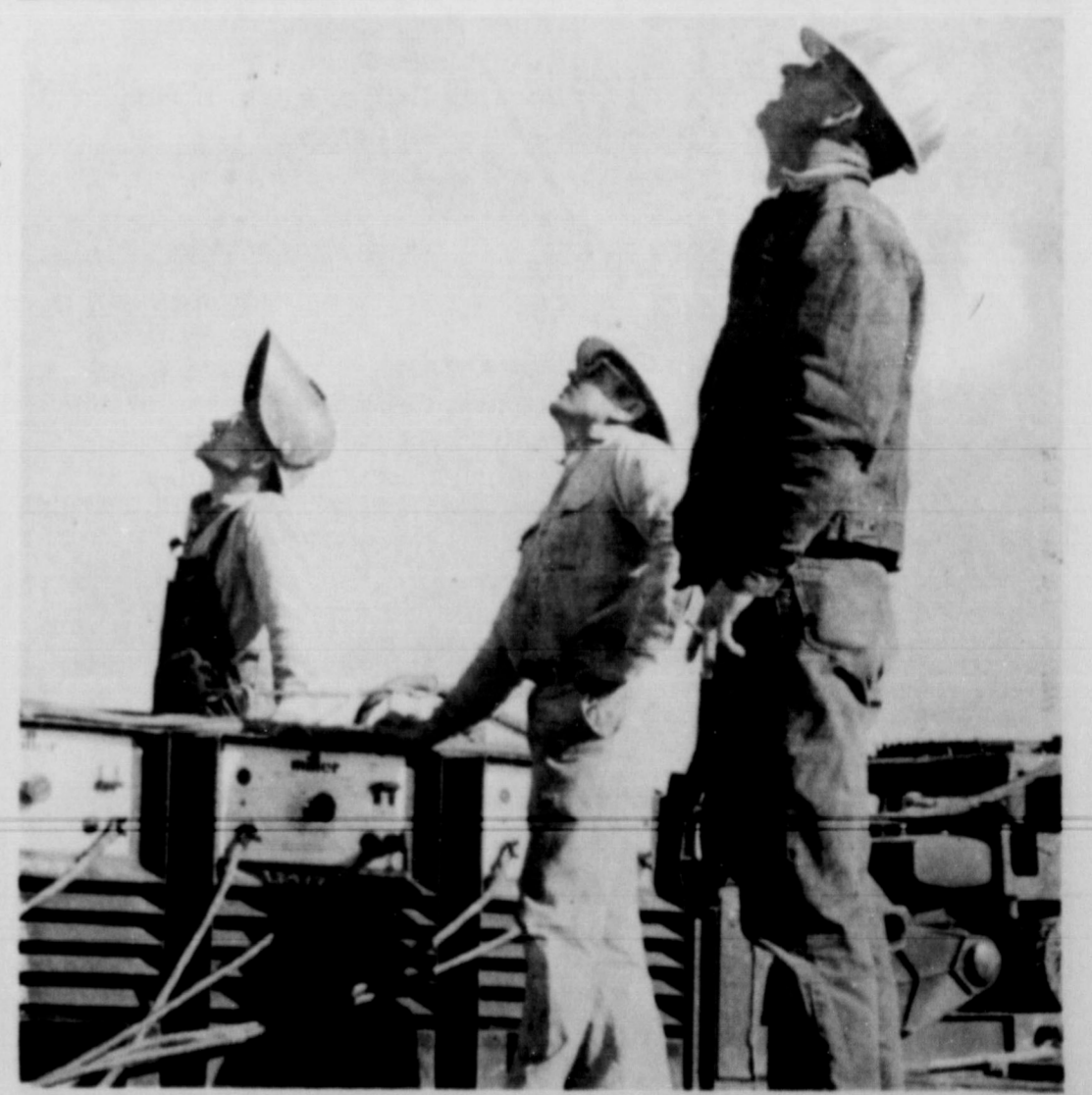
THERE SHE GOES . . . All eyes are on the new water tower project in the northern section of Friona. Construction began in earnest last week, and completion of the tower is expected in a few weeks. This is part of the crew of Chicago Bridge and Iron Company, which is building the tower.
