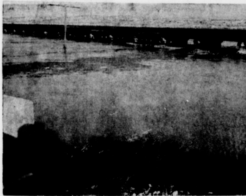
High water Saturday evening in Rankin Draw that crosses Highway 67 about a quarter of a mile east of Rankin city limits, laps at the Santa Fe Railroad Bridge. The bridge has been a victim of the draw's high water on several occasions in the past.
