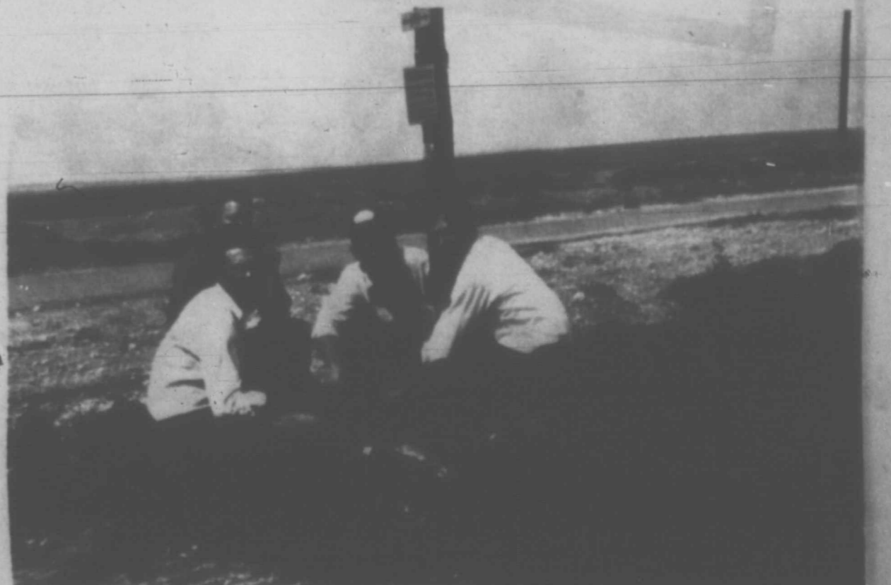
TELEPHONE WORKERS CHECK LINES - Shown above are employees of General Telephone Company at a jack post as they check rural lines which have been converted to 4-party lines. From right to left are Ray Sebring, Had Cantrell, Bill Wells and Jack Rylant. (Staff Photo)
