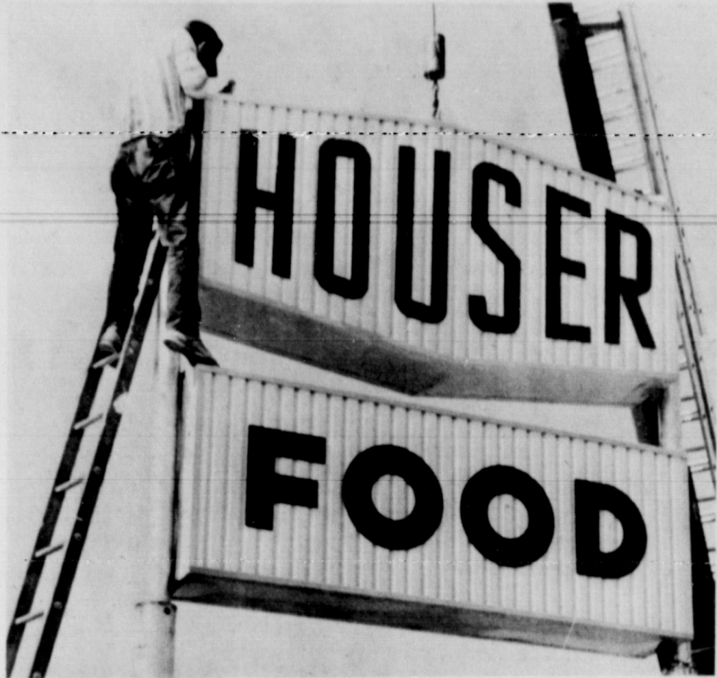
NEW SIGN . . . A workman is shown during the process of installing a new sign for Houser Food Market last week. Housers moved to the location formerly occupied by Piggly Wiggly recently.
