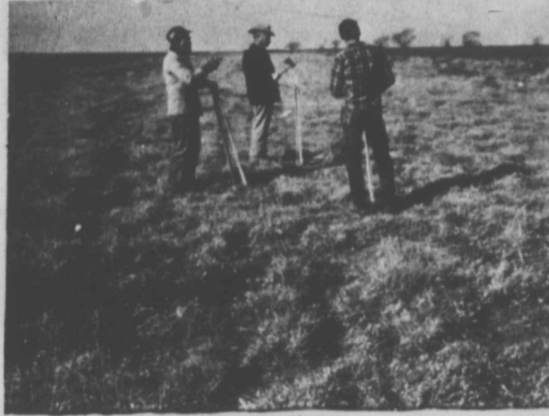
Shown at right are James Withrow with a Soil Conservation Technician and a contractor that are staking the outlet end of a parallel terrace that empties into a constructed and vegetated waterway.
