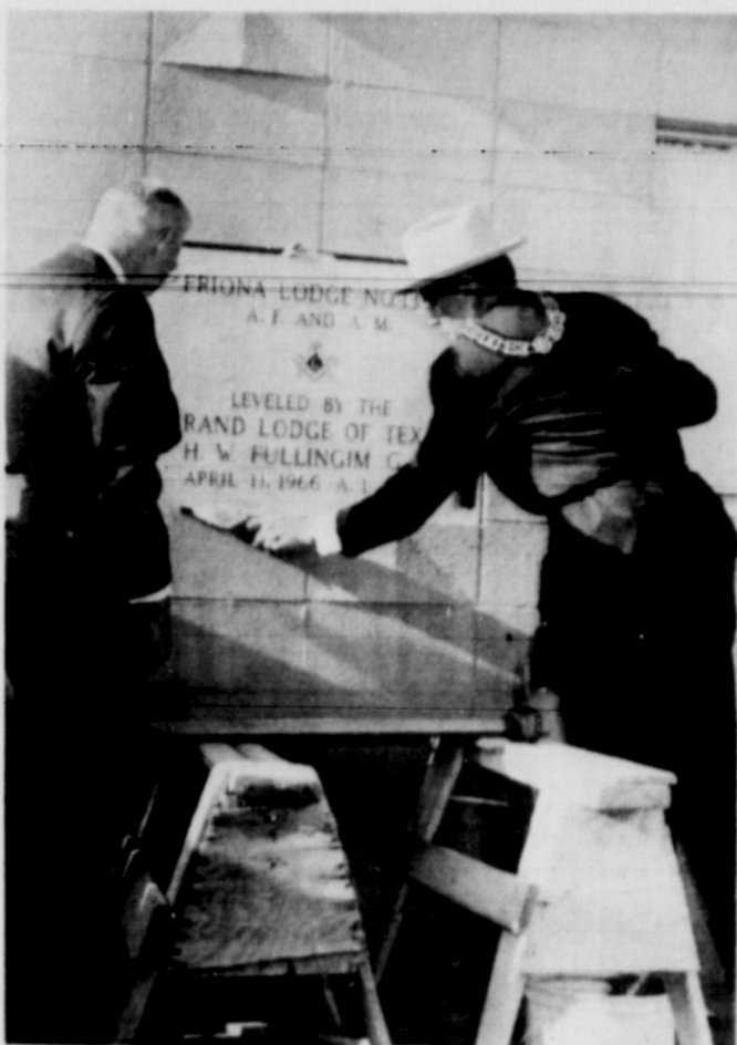
PLACING CORNERSTONE . . . H.W. Fullingim, most worshipful master of Texas Masons, and Lynn Kester, district deputy, are shown setting the cornerstone in Monday's ceremony.
