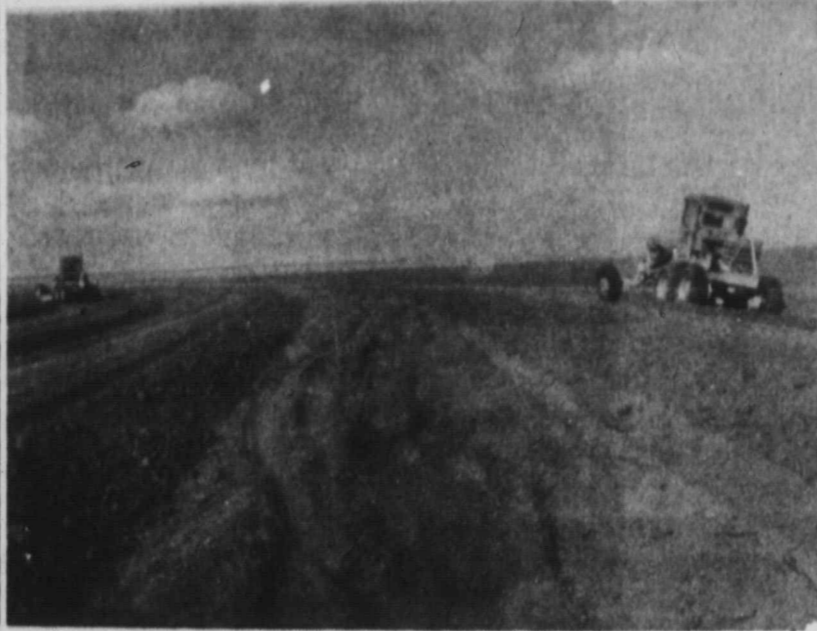
PARALLEL TERRACES BEING CONSTRUCTED AT MRS. NEAL'S FARM, J. C. WITHROW IS THE OPERATOR. SOUTHWEST OF SUDAN. WITHROW STATED THAT AFTER THE HEAVY RAINS THAT WERE RECEIVED ON THIS FARM, THIS YEAR NO DAMAGE WAS DONE.
