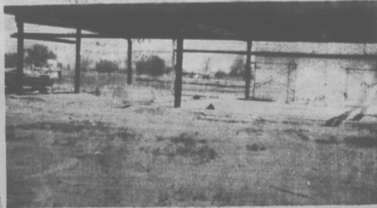
ABOVE IS PICTURED one of the buildings under construction here in Sudan. Chester Irrigation Office is
