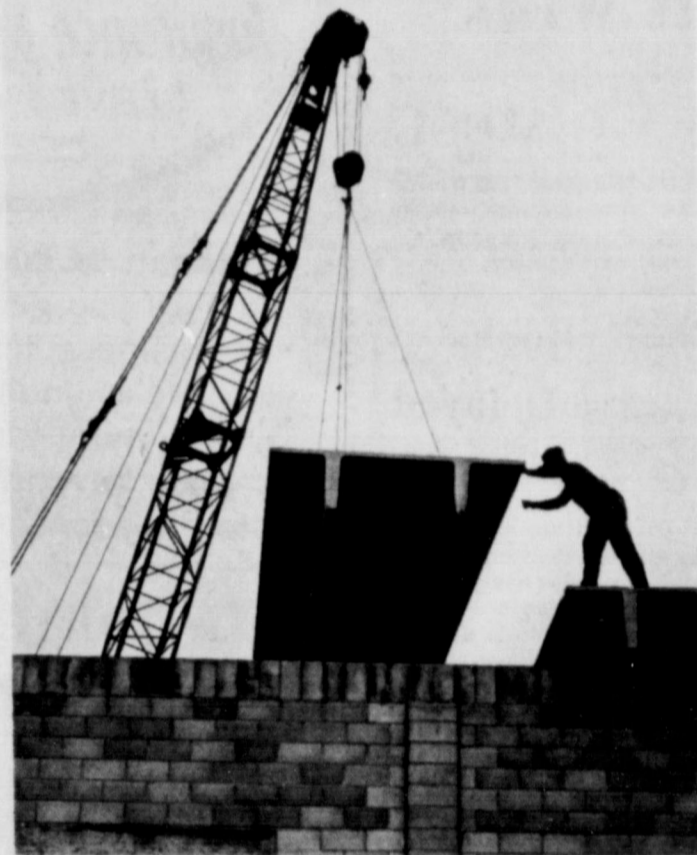
PROGRESS--Concrete beams were recently set in place at Missouri Beef Packers plant southwest of Friona. The plant is expected to be completed in April, 1968. (Staff Photo)
