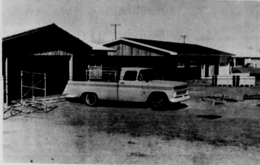
NEW HOMES. . . Shown are two houses under construction by George Taylor on Virginia Street. Building continues at a rapid pace in Friona with several new permits issued since the first of the year.
