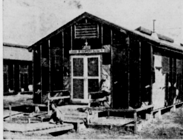
CROWDED AND FALLING APART are many of the buildings at the Mexia State School, shown above, which houses the young feeble-minded of the State and senile men and women. The picture above shows a group of patients crowded on a porch (an attendant is in the foreground) because they have no other place to sit. Below, is one of the old tar-paper shacks at Mexia, which in 1943 was used to house war prisoners. The photo shows how it is falling apart at the seams, yet it is still being used to house mentally deficient children.
