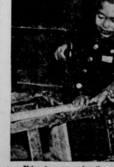
Using hammer and nails sent by the American Junior Red Cross, school boys at Sung Buk Primary School, Seoul, repair school furniture. The carpentry materials were part of a school assistance unit, one of a thousand sent last winter to help rebuild and repair schools in Korea.
