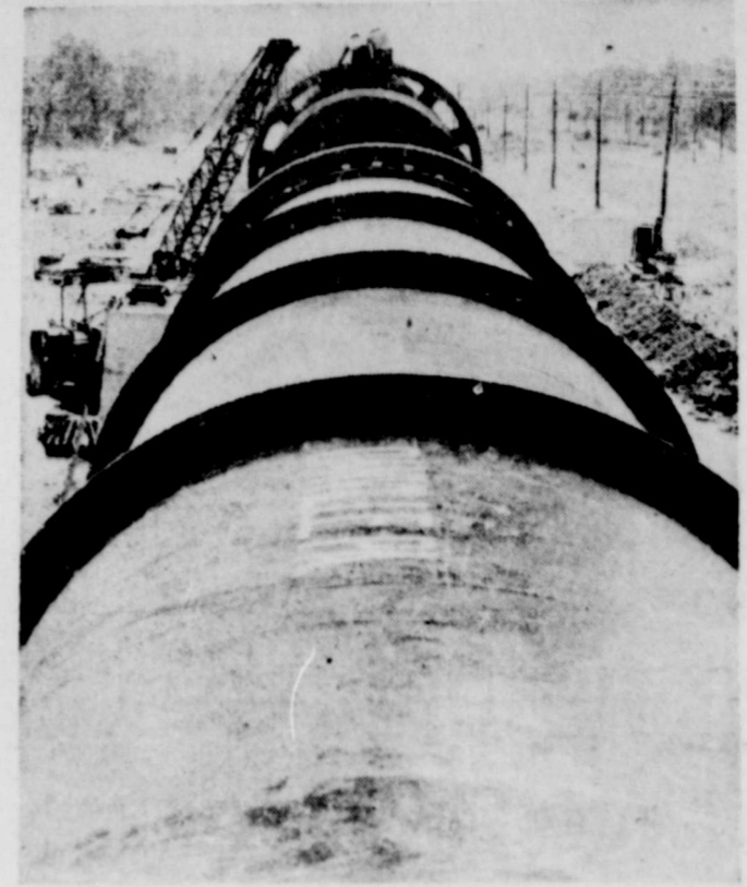
One of the world's largest single pieces of precision mechanized equipment, a 300-foot rotary kiln for the manufacture of cement, is being completed at the Texas Portland Cement Plant at Orange, Texas.
