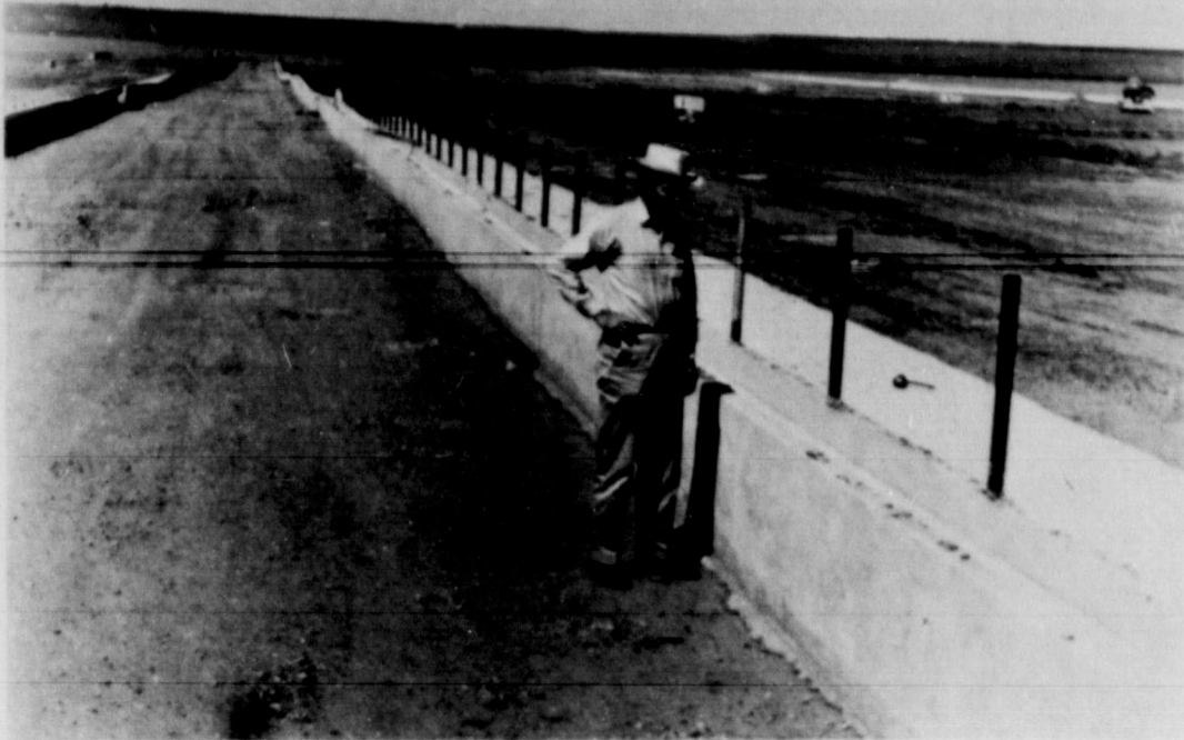
FEEDLOT SITE. . . A.L. Black surveys work going on at the new feedlot site south of Hub. Much water and concrete work has already been done, as evidenced by the concrete bunkers in the picture, the new lot which hopes to open in November, will have a capacity of 20,000 head.
