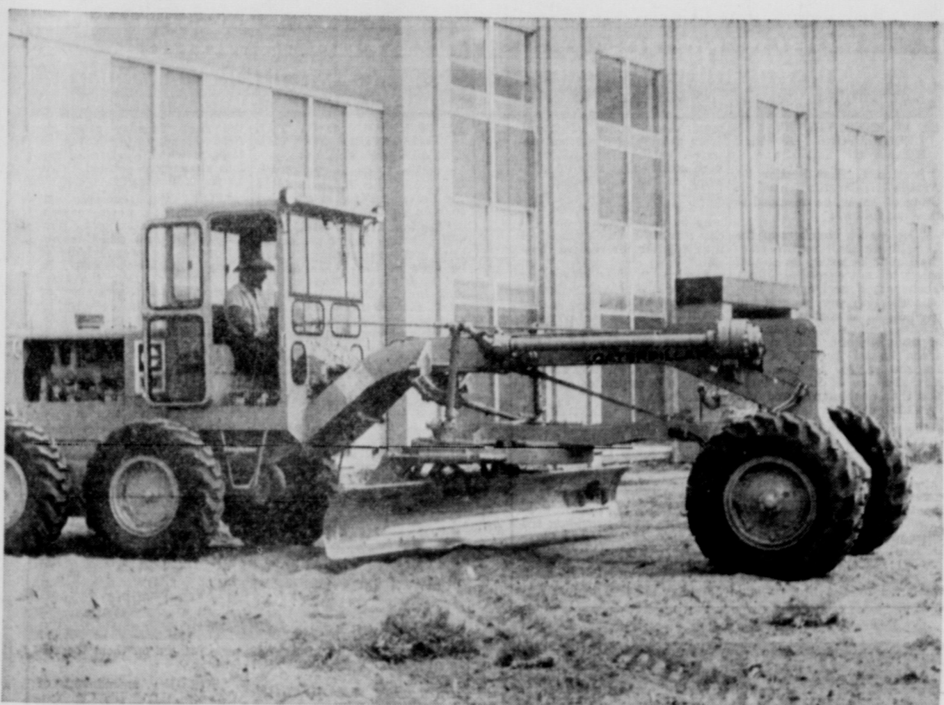
Final clean-up . . . GROUND WORK around the newly remodeled Cochran County Courthouse was completed this week. This was the final phase of the remodeling, the inside having already been completed.
