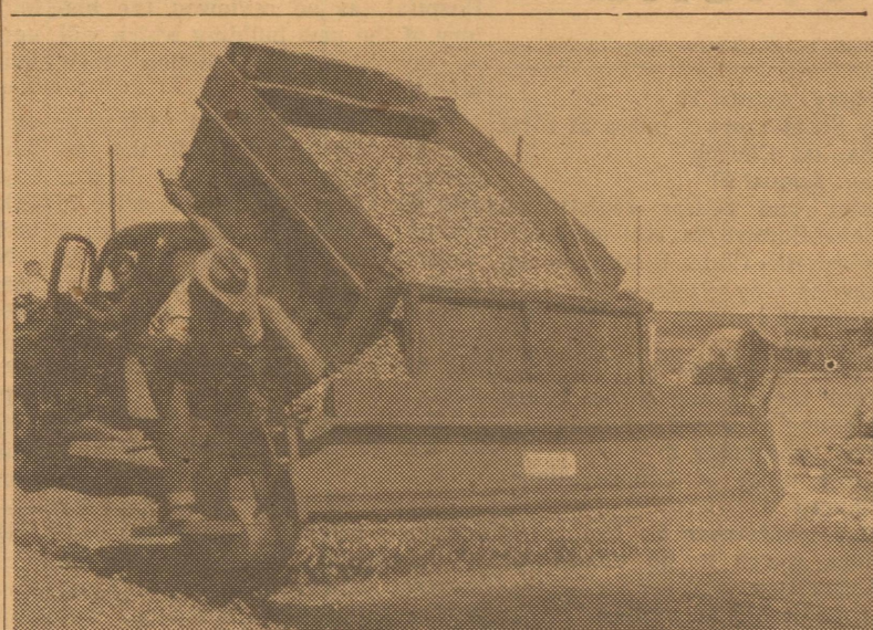
HALLELUJAH!—That's what Friona residents are saying at the sight of asphalt topping finally going down on the Highway 60 widening project through town. Here a dump truck spreads gravel in the first stage of the topping.
