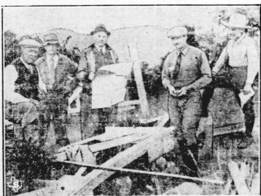
Here are the first views of construction work just begun atop Mount Locke, Davis Mountains of West Texas, on the Mount Locke Astronomical Observatory, which will be the second largest in the world. In the picture are several members of the construction company which will build the observatory, and at the right is Prof. G. Van Biesbroeck, astronomer of the Yerkes observatory, who will orientate the building with the stars. The observatory is being built by the University of Texas and the University of Chicago.
