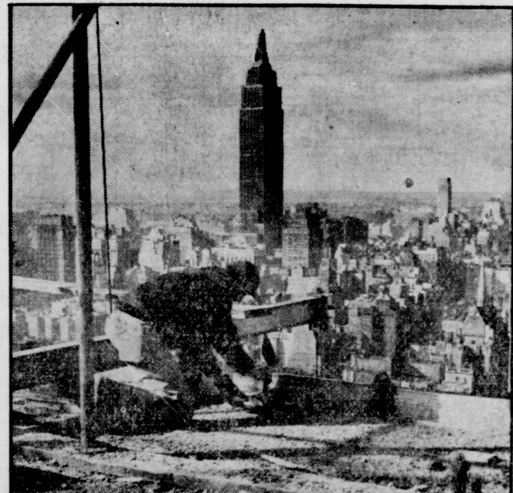
NEW HORIZON SHAPES UP — This workman, high above Franklin D. Roosevelt Drive in New York on the 42-story UN Secretariat Building, has to himself a view which will soon be admired by world planners. The Empire State Building dominates the view.
