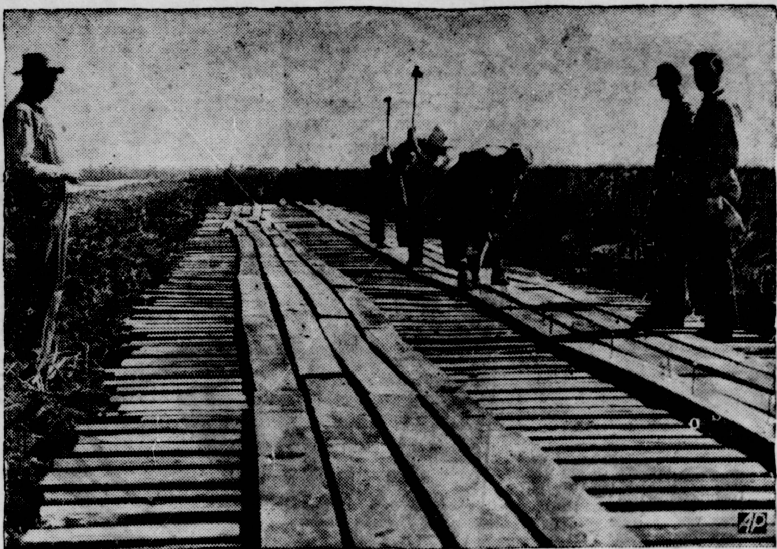
HARDWOOD HIGHWAY —Workmen are "hard-surfacing" a mile-long road from US Highway 90 to a new oilfield in the marsh- es near Orange, Tex. Thick oak boards laid on top of a roadbed dredged out of the marsh will bear the weight of big trucks and machines to be moved in to develop the oil field. The hardwood highway is being constructed by Ohio Oil Co., which discovered the new field. (AP Wirephoto)
