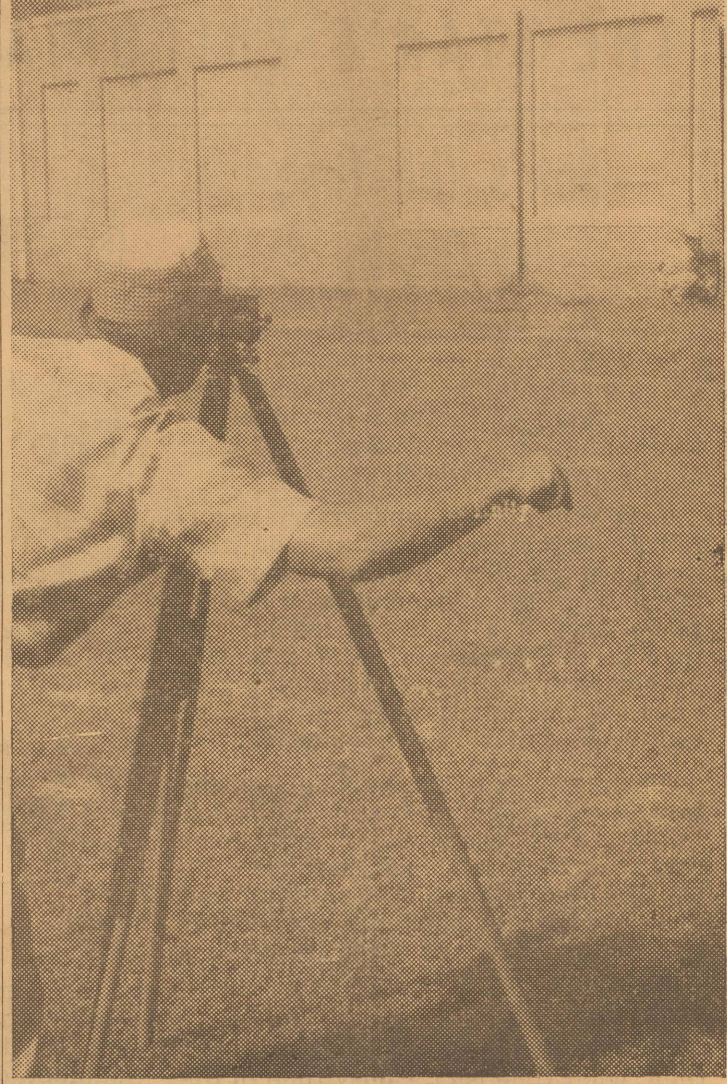
"DOWN A HAIR—and that will get it." Workmen are checking ground elevations to see how much levelling will be required to pour foundations.
