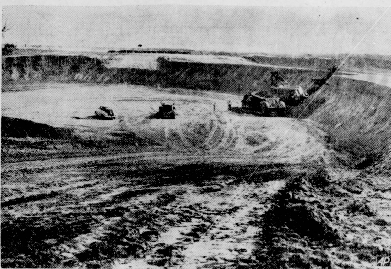
Earth moving machines continue work on the international Falcon dam being constructed on the Lower Rio Grande near McAllen. Except for spillways and power plants in the river bed, the five-mile-long structure is earthen. (AP Photo).
