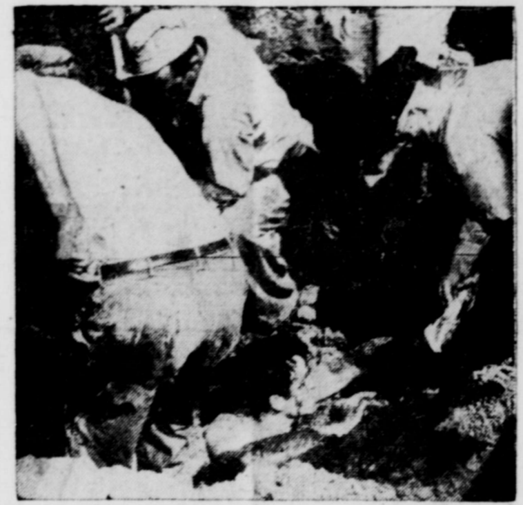
Workmen dig frantically to release Donald Cooper, 22, as Capt. Arthur Moran of the Omaha Fire Dept. rescue squad put splints on Cooper's broken finger. Buried under five feet of dirt for almost 15 minutes when a bank caved in on a sewer project, Cooper's only injury was the broken finger. (NEA Telephoto).
