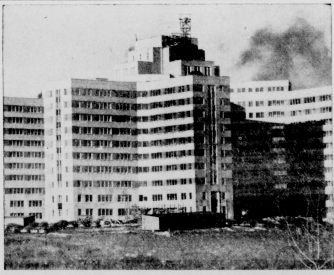
NEARING COMPLETION—The outer shell of the new Veterans' Administration Hospital, in Albany, N.Y., is almost finished. The 14-story building, of fireproof construction, will have a capacity of 1000 beds when it's ready for the first patients.
