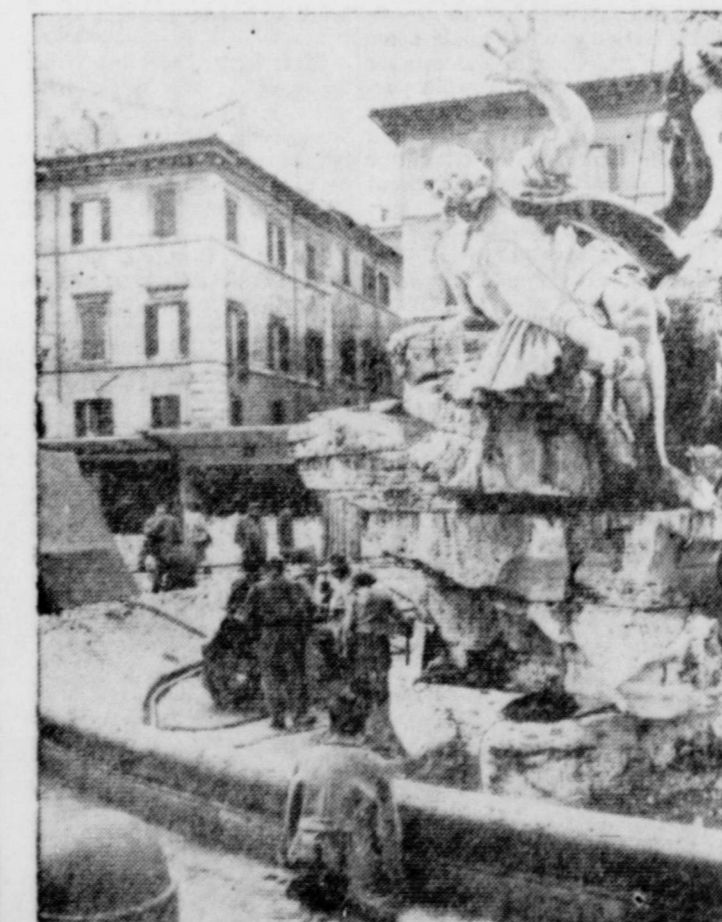
DRIED FOR REPAIRS —The basin of the famed Piazza Navona Fountain in Rome was dried so workmen could repair a broken pipe. The work of Italian sculptor Lorenzo Bernini, the fountain represents the four longest rivers in the world. The huge statues which adorn the fountain dominate one of the most beautiful squares in the Eternal City.
