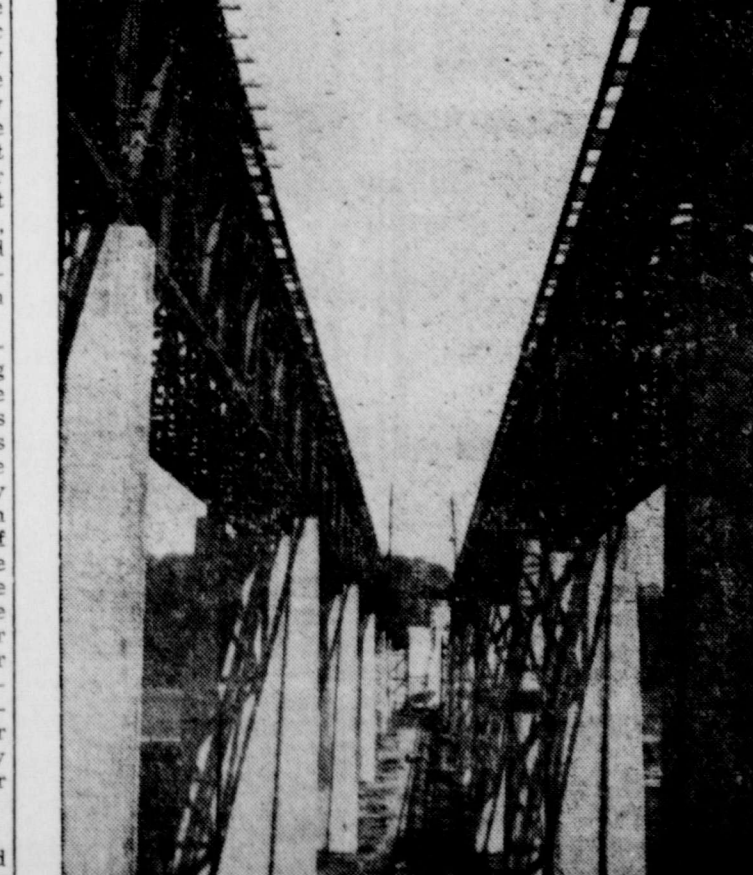
SOME TIME NEXT YEAR—Concrete, steel and sky make an interesting contrast as these two bridges are constructed over the Cuyahoga Valley at Peninsula, O. The twin spans are part of the new turnpike being built across Ohio. One end of the 241-mile stretch is connected to the Pennsylvania Turnpike, and the other ends in a pasture at the Indiana border. The $326,000,000 project is scheduled for completion on November 1, 1955.
