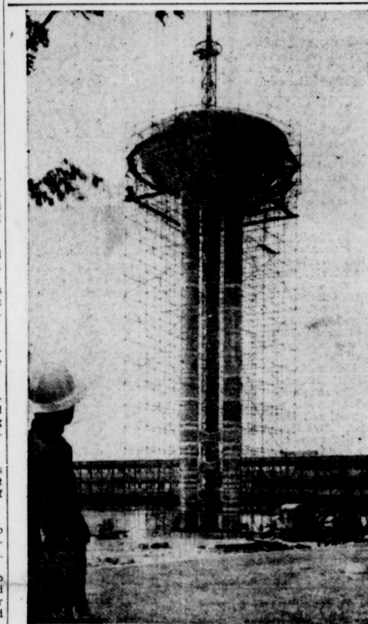
WAITING FOR ITS TOPPER—The lower half-shell of a 250,000-gallon stainless-steel-clad water tower rises skyward at the General Motors Technical Center in Detroit. When the upper half is placed on the tower it will bring the structure's total height to 132 feet. Three steel columns, each six feet in diameter, support the tower.
