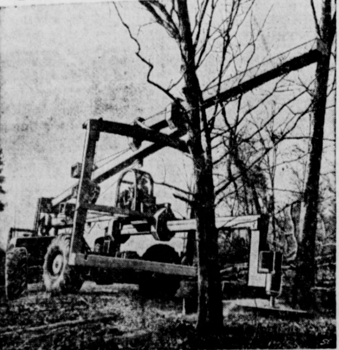
A newly-designed mobile saw is here shown felling a large tree in a 16,000-acre land clearing project near Texarkana, Texas. One man sitting comfortably in a protective steel cage and operating simple controls moves the huge apparatus up to a tree from any angle and within seconds has it crashing to the ground. The unit, designed by R. G. Le Tourneau, Inc., of Longview, Texas, is electrically operated, producing its own current by means of a generator driven by a General Motors Diesel engine.
