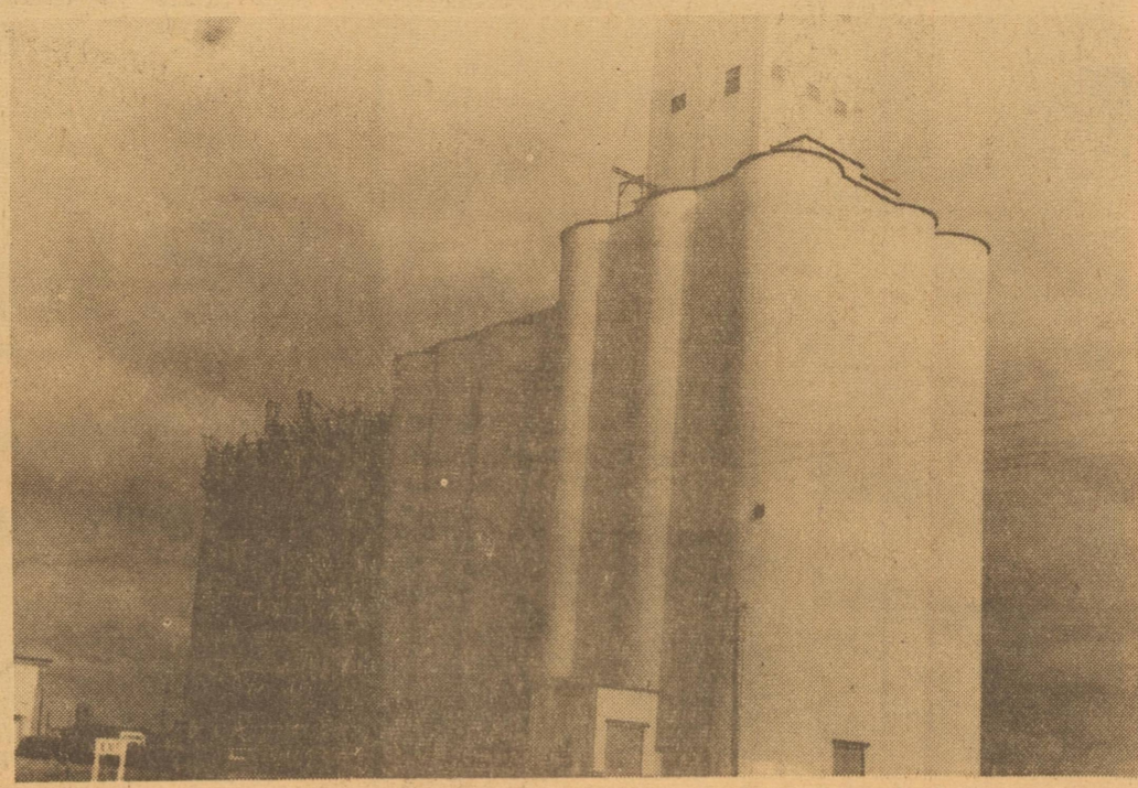
UP, UP go steel and concrete to swell Parmer County's ever increasing capacity to store grain--still the biggest crop grown here. This addition is to the Sherley-Anderson-Pitman elevator in Farwell. One sad note on this otherwise good news; a workman was killed in a fall from the construction site Sunday night.
