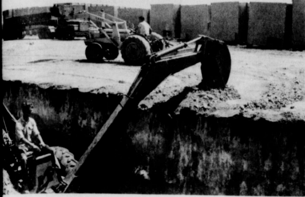
Like a Dinosaur of the deep, a mechanical shovel prepares the foundation for 14 bunker feed mill, at Hansford Feed Yards, near Spearman.
