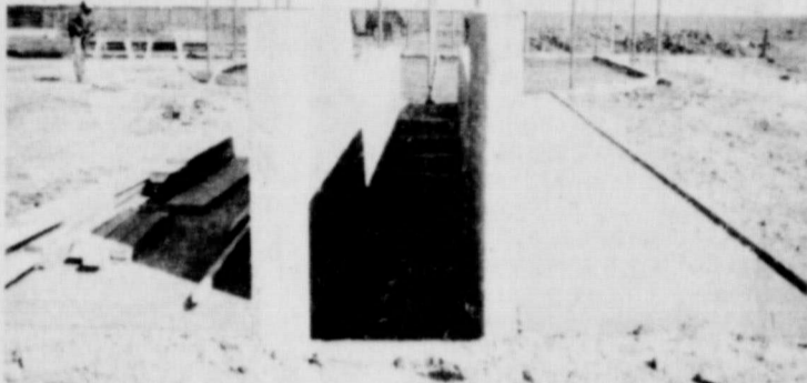
MUCH OF THE CEMENT work for the cattle dipping vat now under construction on the Dee Allen farm south of Spearman has been done. This public facility will be completed in the near future. The State is requiring this type of dipping facility for the control of scabies.
