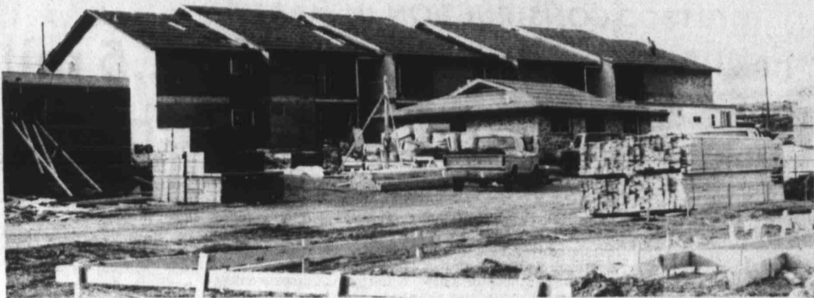
MORE APARTMENTS — These apartments, being built by Heinze Construction on Wasson Road, already have a waiting list of eight tenants. The demand for more apartments and houses has been heavy in the Big Spring area during the past year.
