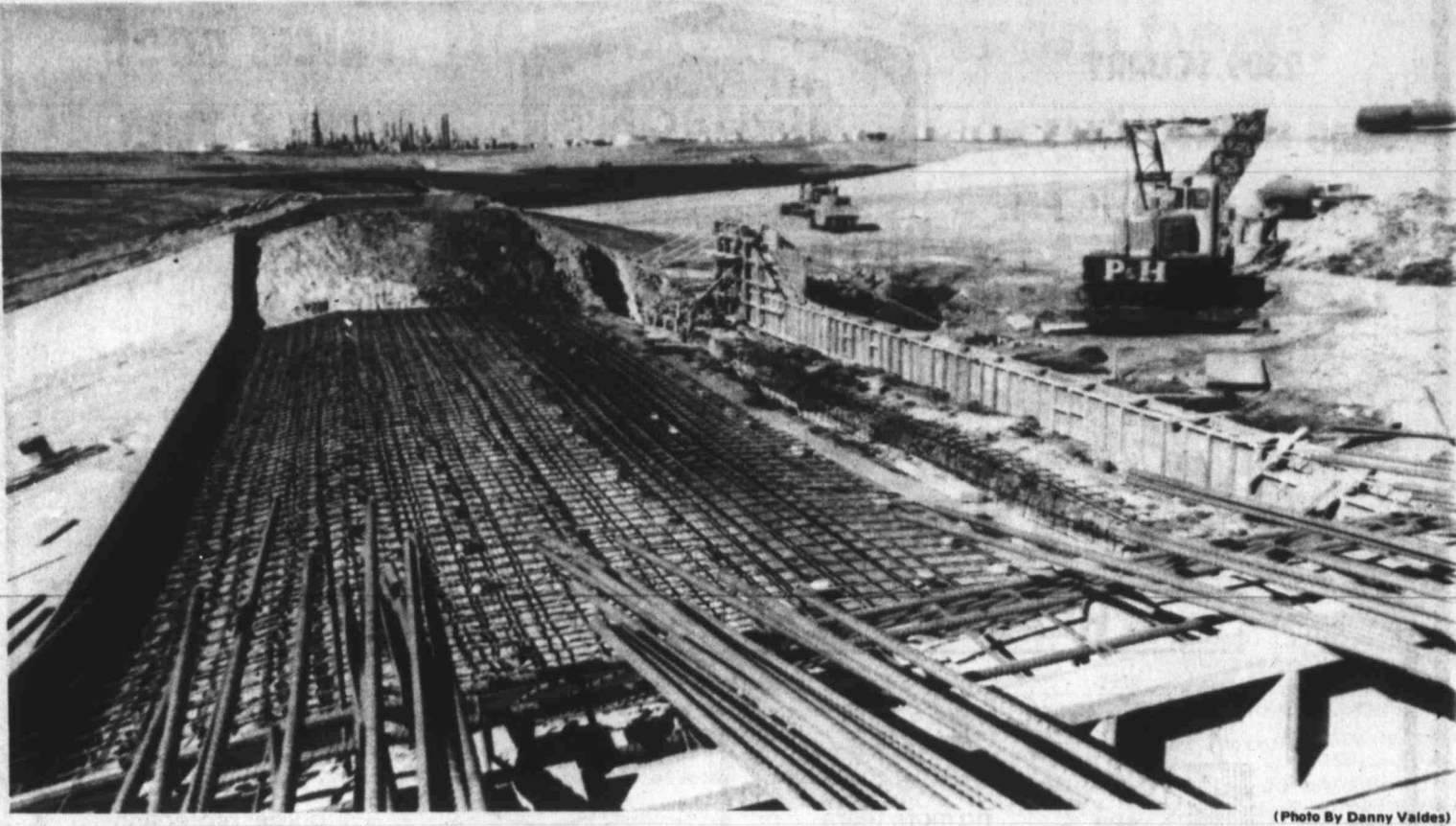
FOR SPEEDY RUNOFF — The new Cosden Lake being constructed by Cosden Oil and Chemical Company will transform the rough terrain into a lake designed to hold surface runoff and wastewater from the complex.
