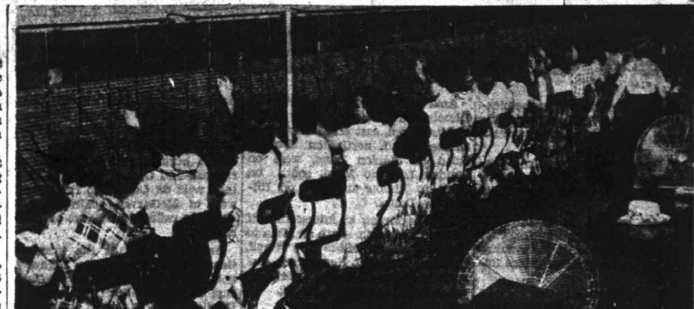
FLASHING LIGHTS —This is the manual switchboard at the Midland telephone office which handles 68,000 local and 3,000 long distance calls a day. Telephone operators' hands constantly are plugging in or pulling out the plugs on cords that connect callers with their numbers. With all plugs busy the callers' lights flash to no avail until a line is free.
