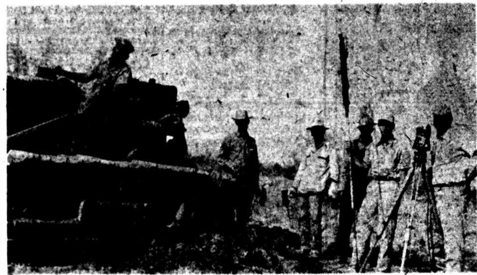
WORK UNDER WAY —Clearing land of brush and preparing sites for construction of Phillips Petroleum Company's new gasoline plant in the Spraberry Trend in Midland County, Texas, is under way. One of the bulldozers is shown here clearing ground for the first construction. R. C. Pickles, right, and H. M. Faulconer, Phillips engineers, are shown at the transit. Bulldozer operator is V. L. Conatser.
