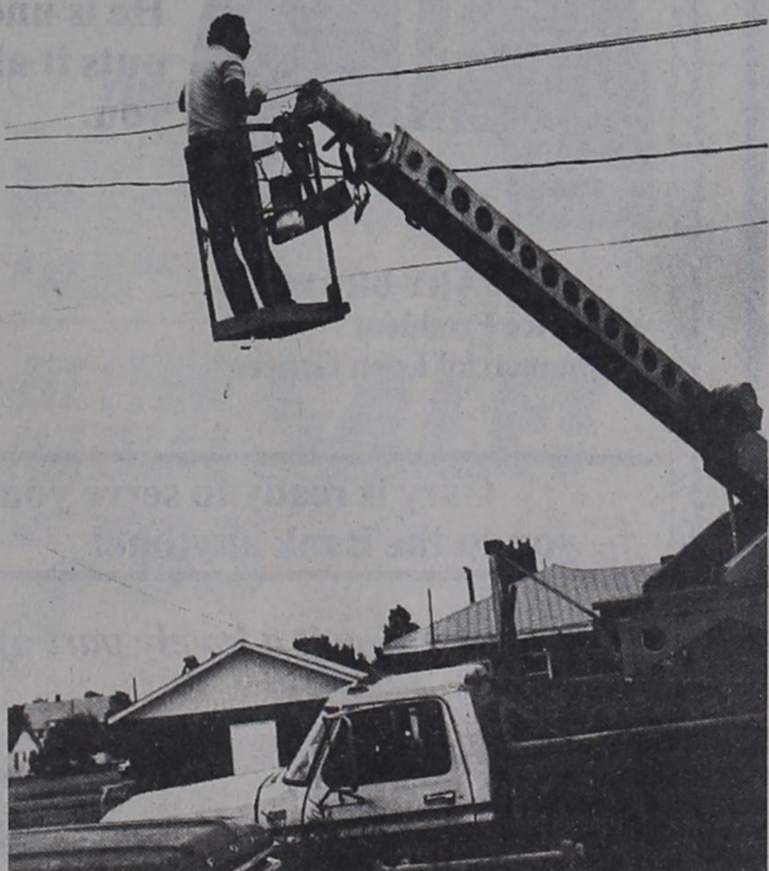
'PHONE REPAIR... If you tried to call a business in the 900 block of Main Street or Washington Street Thursday morning, you couldn't get them, because every telephone in the square block was out of order to begin the day. General Telephone Company's repairman is shown making the repairs.
